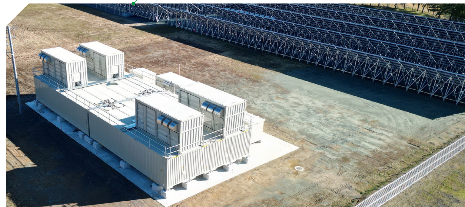
Redox flow battery and solar panels installed in Kashiwazaki City, Niigata Prefecture, as a grid-scale storage system for a new regional power utility. With an output of 1,000kW and a capacity of 8,000kWh, this large-scale facility can provide approximately 8 hours of discharge, making it one of the longest-duration systems in Japan.
