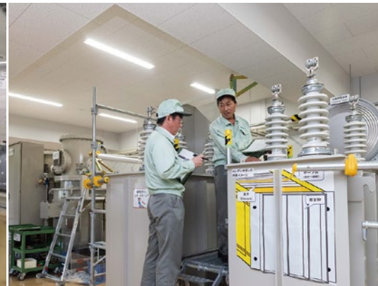
Veteran engineers certified by the company as Meisters take the lead as instructors for hands-on training using actual equipment, such as substation equipment operation, maintenance, and inspection, helping to ensure the transfer of technical expertise.
