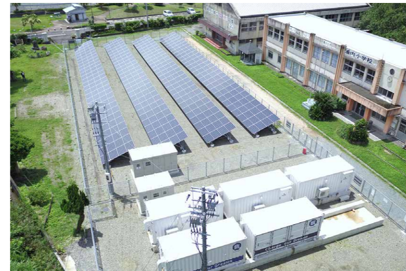
Koshikishima Urauchi Solar Power Plant with max. 100 kW output and Koshikishima Storage Battery Center housing storage batteries removed from 36 Nissan Leaf EVs were constructed on the grounds of a former elementary school (top). These facilities came on stream in 2015 and the municipality is scheduled to start a project in 2018. The inside of a container at the storage battery center (left). Storage batteries previously used for EVs are installed on partitioned racks.
